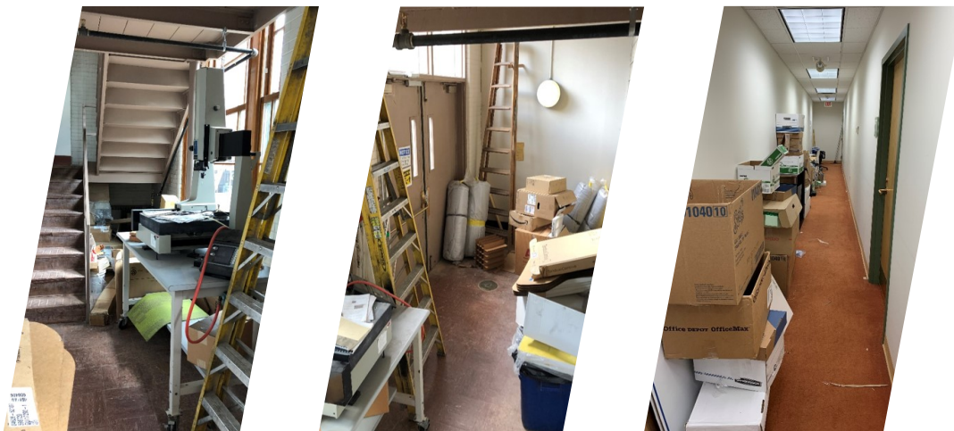
Examples of obstructed egress
