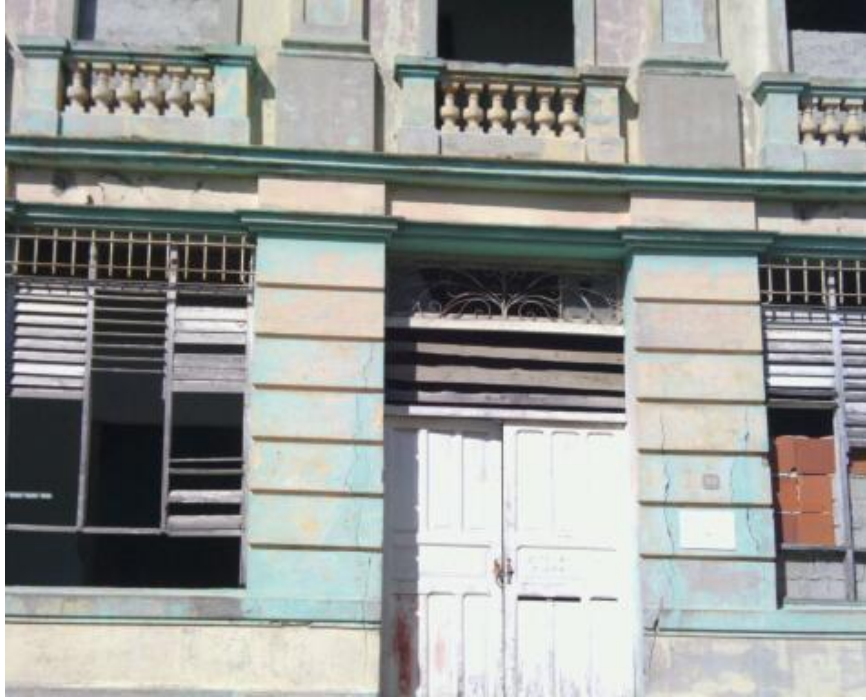
Polyclinic on Martí and Aguilera Streets, in danger of collapsing, with its workers spread out over the entire city in small locales, or abroad helping other countries.
