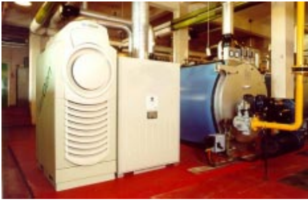
A 30-kW microturbine provides heat and power for a municipal building in Durham, England. Photo courtesy of Capstone Microturbines.
