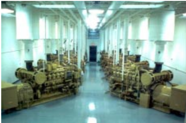
Eight 800-kW Caterpillar engines supply power to a plastics plant in Illinois. Design and photo by LaSalle Associates.
