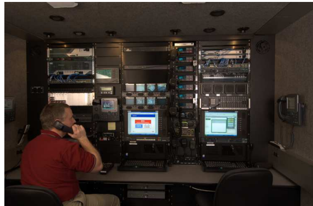
Figure 2: The engineering section of the Cisco NERV brings together different technologies to provide situational awareness for the command staff.
