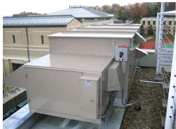
Energy Wheel System Installed at the CMU IW
