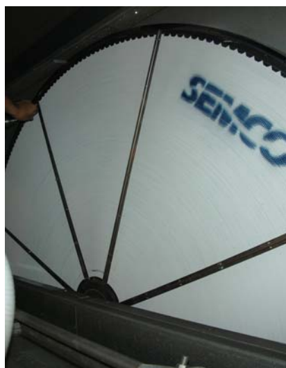
New 3 Angstrom Media Installed
