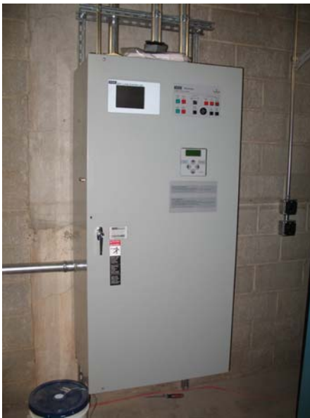
Figure 7. Soft Load Controller (SLC) and Automatic Transfer Switch (ATS)
