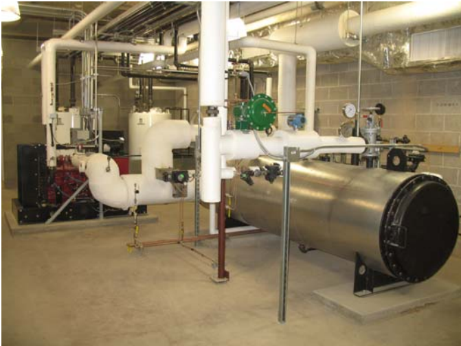
Figure 4. Biodiesel Fueled Engine Generator with Heat Recovery System
