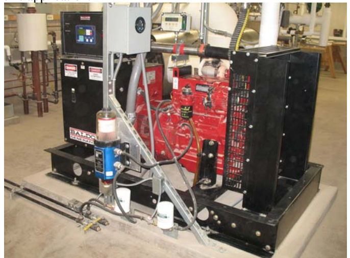
Figure 6. 25 kW Engine Generator Set
