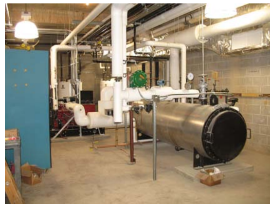
BioDiesel Engine Generator with Heat Recovery Equipment in MMCH C9
