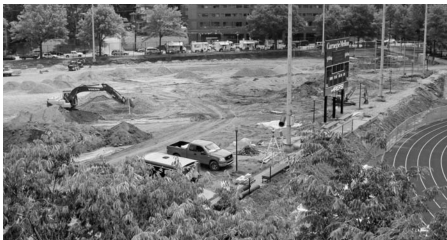
A REGULATION-SIZE SYNTHETIC SURFACE SOCCER FIELD IS BEING BUILT ON THE INTRAMURAL FIELD. THE PROJECT WILL REDUCE MAINTENANCE COSTS TO THE AREA.
