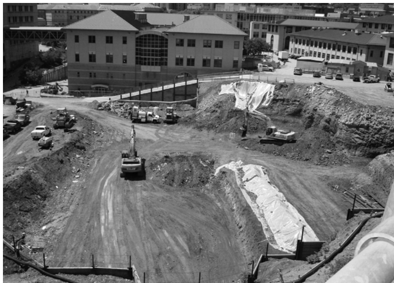
BY THE TIME STUDENTS RETURN TO CAMPUS IN AUGUST, THE CONSTRUCTION SITE FOR THE SCS COMPLEX WILL SPORT CONCRETE PILLARS FOR THE 150-CAR SUBTERRANEAN GARAGE.
