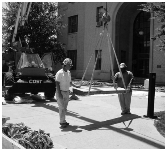
DOHERTY HALL WILL GET A FACELIFT THIS SUMMER, AS THE STAIRS AND FRONT ENTRANCE WILL BE REDONE.
