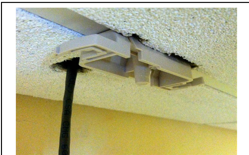
Cutting of ceiling tiles to allow tiles to reseal properly for Tegular ceiling tiles.
