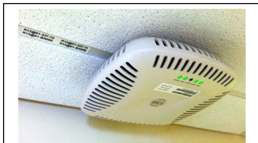
Correct outlet labeling on drop ceiling rails and correct orientation of Aruba AP with LEDs facing away from wall.
